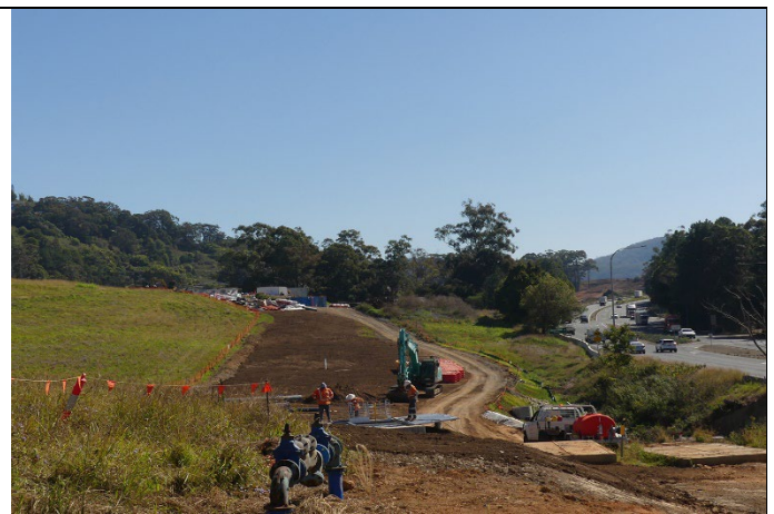
More construction work making one of the ramps, south of the Bruxner Road turn off.
