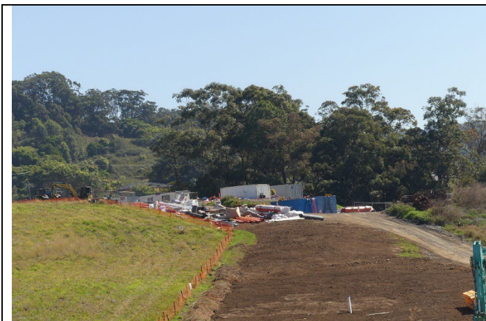
Construction work on the western side – just past the Bananacoast Caravan Park.
